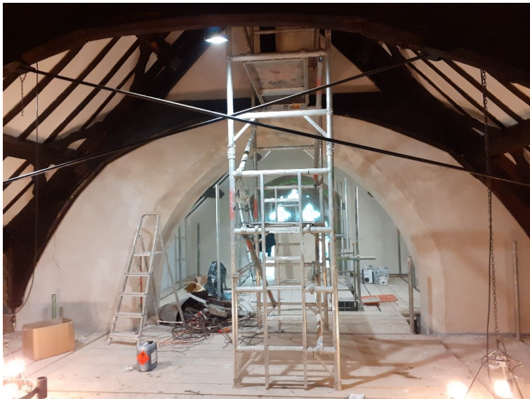
Plaster not yet dry to East and West ends
